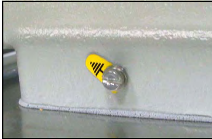
Figure 29: Earth Ground Connection
